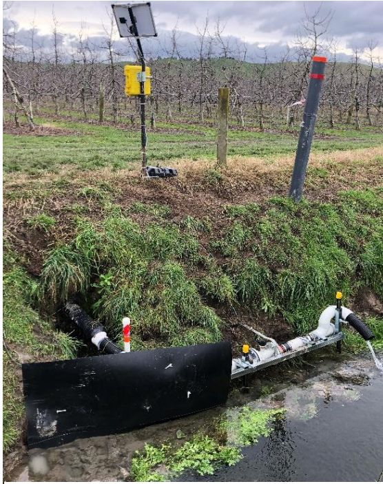
Figure 8 In Drain Proportional Sampling and Flow Metering equipment
