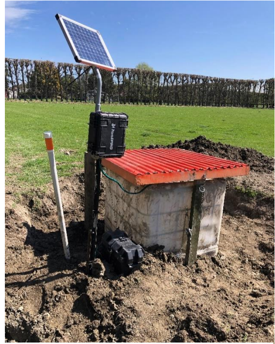
Figure 7 Pod Proportional Sampling and Flow metering equipment
